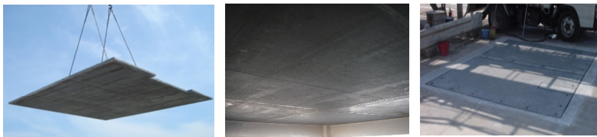
Photo 1 Application of EIEN. (L-R) Buried form of EIEN, repair of pier soffits using buried form, protective layer upper surface of pier
